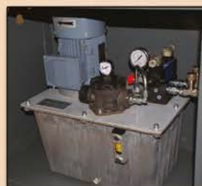
Centralina griglia mobile Moving grate oil gearcase
